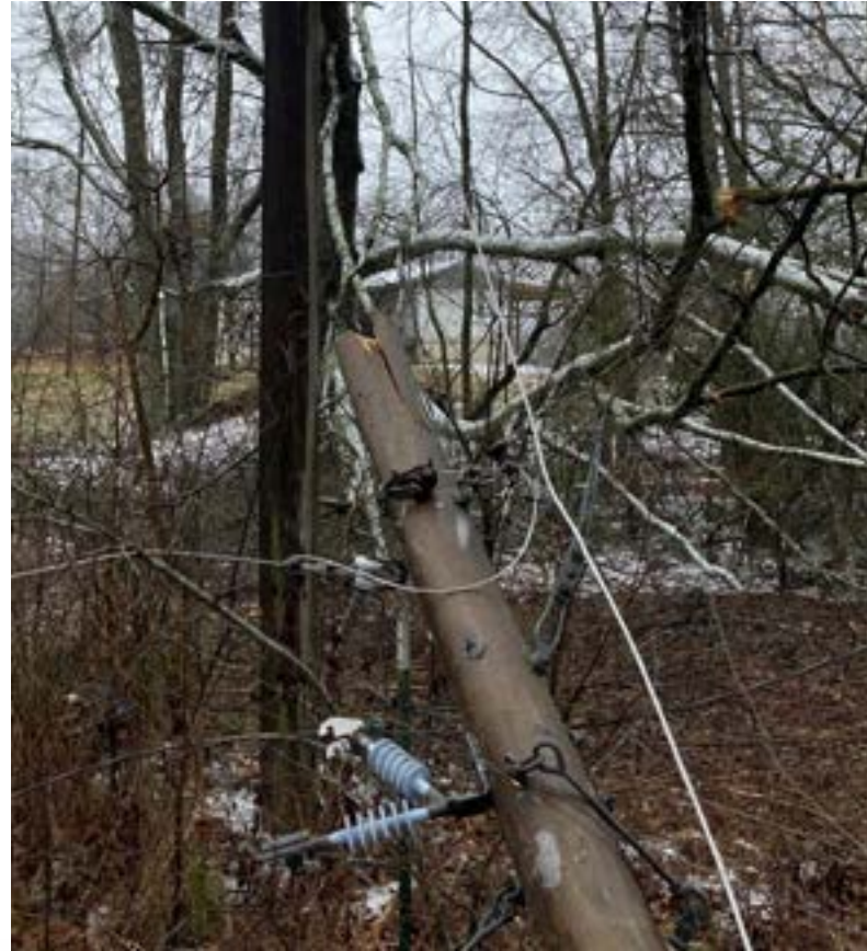
The damage to our electrical system was extensive due to the ice.
