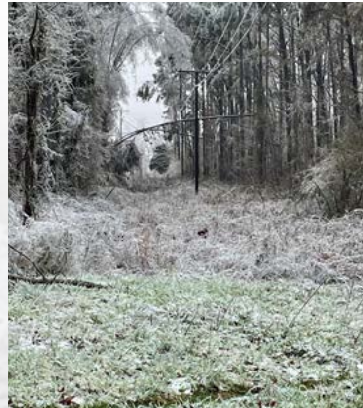
Many trees could not bear the weight of ice and fell on power lines.
